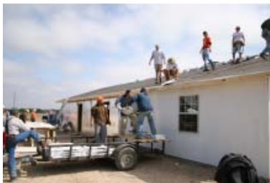
Construction team members build a dining hall/kitchen for an orphanage in Morelos, Mexico
